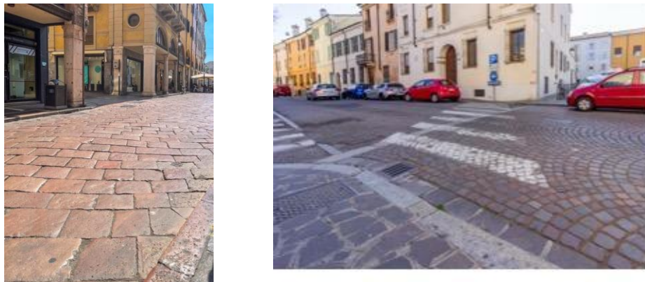
Figure 50 - 51. City of Mantua. In the image on the left, a street in the pedestrian area of the historic centre; the pavement is in low maintenance condition, with numerous depressions and discontinuities, posing a risk of falling. On the right, a pedestrian crossing extending diagonally, which lacks tactile pavement for orientation, making it difficult for blind and visually impaired pedestrians to identify it and navigate it safely (Sebastiano Marconcini, 2025)
