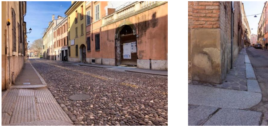
Figure 46-47. City of Mantua. The sidewalks, throughout its entire length or in specific areas such as driveways, present excessive cross slopes. This creates a risk for individuals using mobility aids, making it difficult for them to navigate safely and comfortably (Sebastiano Marconcini, 2025)
